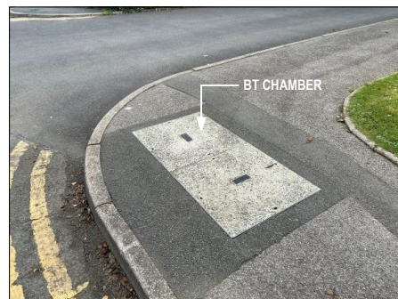
PHOTOGRAPH 2 EXISTING BT CHAMBER ON THE WILLOWFORD ADJACENT TO JUNCTION WITH MAIN AVENUE
