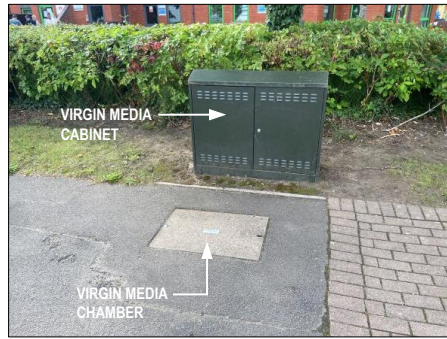
PHOTOGRAPH 5 EXISTING VIRGIN MEDIA CABINET AND CHAMBER IN FOOTWAY ON MAIN AVENUE ADJACENT TO BUILDING
