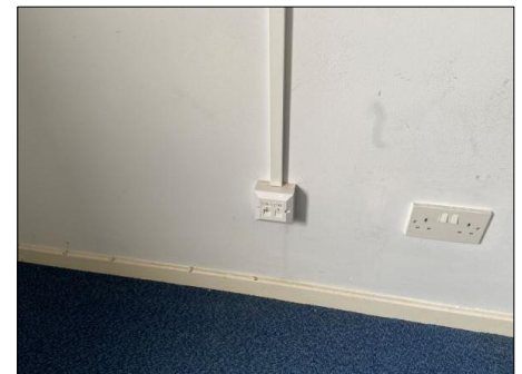
PHOTOGRAPH 12 TYPICAL VIEW OF EXISTING TELECOMS OUTLETS LOCATED ON FIRST FLOOR
