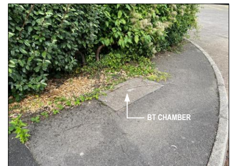
PHOTOGRAPH 3 EXISTING BT CHAMBER IN FOOTWAY ON THE WILLOWFORD TO NORTH OF BUILDING
