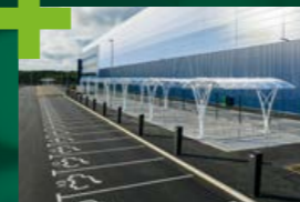
Fast car charging (EV)
